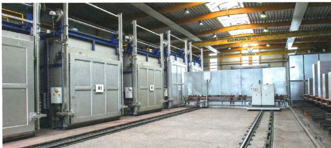
Fully automatic plant for heat treatment at Gleich
